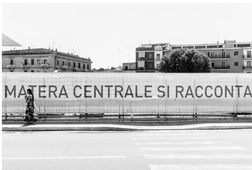
Figure 1. Work in progress for the new station FAL Matera Centrale, July 2019. (Photo by Ciriaca Coretti)
